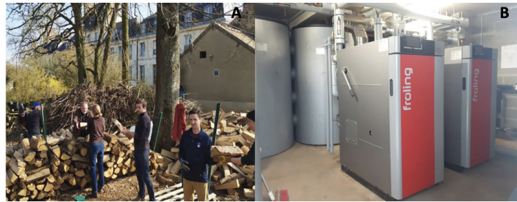
Figure 8. Wood stock (A) at the Campus and the two wood-fire boilers (B)
